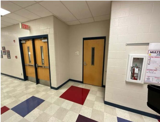
31 - FIRE EXTINGUISHER AND ALARM DEVICE
