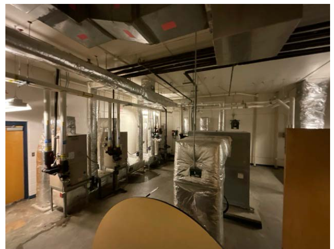
24 - SECONDARY MECHANICAL ROOM
