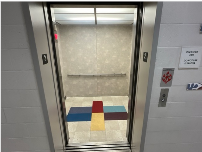
LOBBY LOOKING AT CABS (WITH DOORS OPEN)
