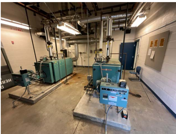
23 - MAIN MECHANICAL ROOM
