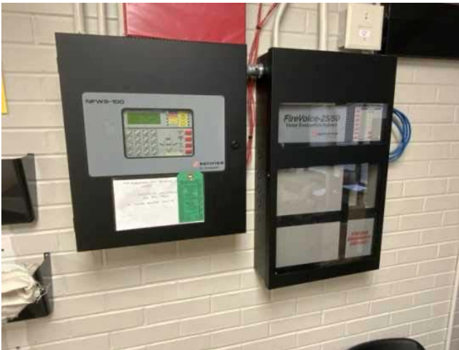
27 - FIRE ALARM PANEL
