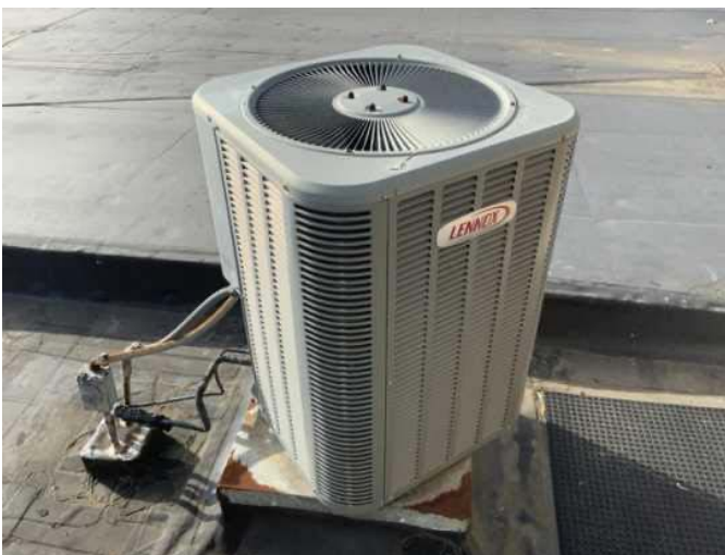
17 - SPLIT SYSTEM HEAT PUMP
