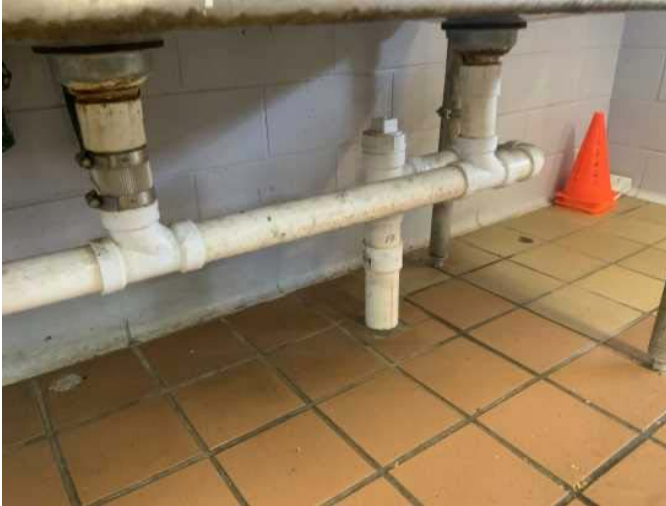
13 - PLUMBING SYSTEM PIPING
