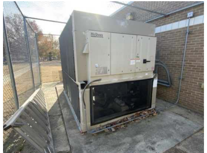
16 - AIR COOLED CHILLER
