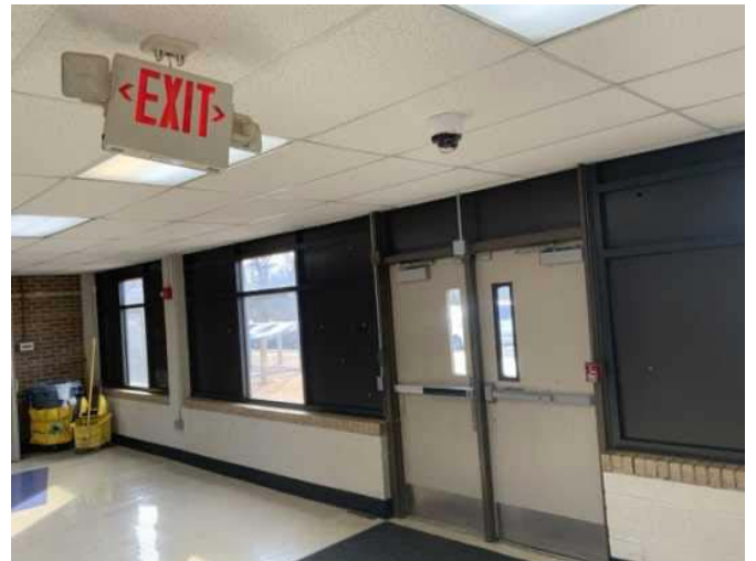
28 - FIRE ALARM SYSTEM COMPONENTS
