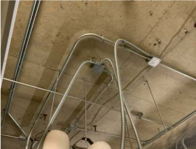
25 - ELECTRICAL SYSTEM WIRING
