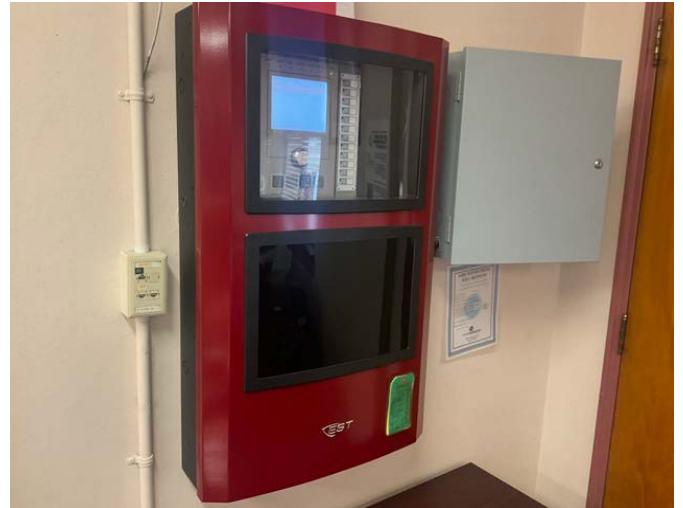
20 - FIRE ALARM PANEL
