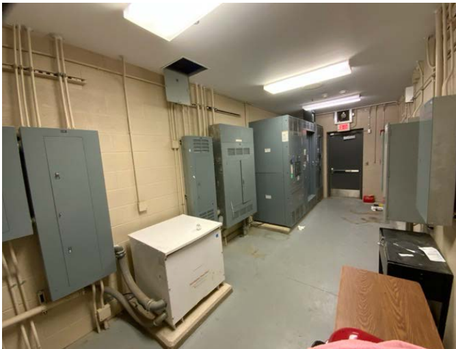
27 - MAIN ELECTRICAL ROOM
