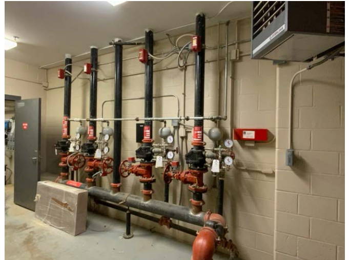
26 - FIRE PROTECTION ROOM
