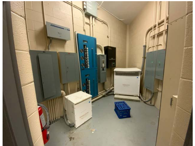
28 - SECONDARY ELECTRICAL ROOM
