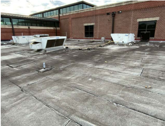
25 - ROOFTOP MECHANICAL EQUIPMENT
