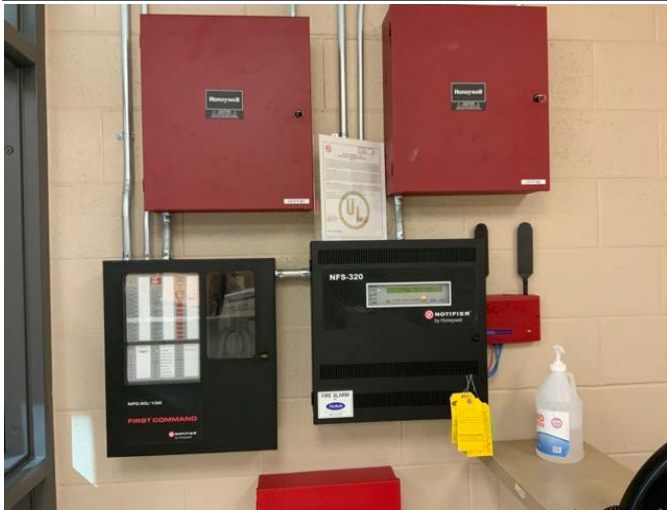
31 - FIRE ALARM PANEL
