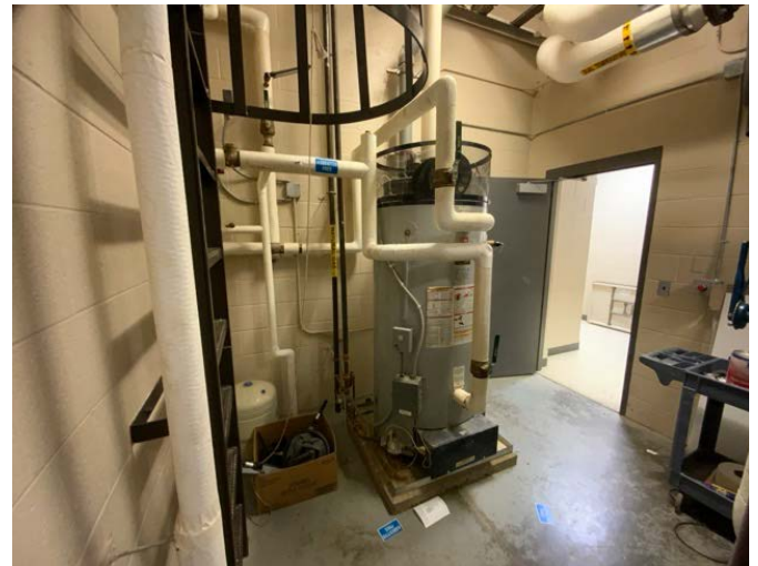
22 - DOMESTIC HOT WATER SUPPLY
