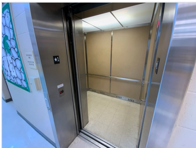
LOBBY LOOKING AT CABS (WITH DOORS OPEN)
