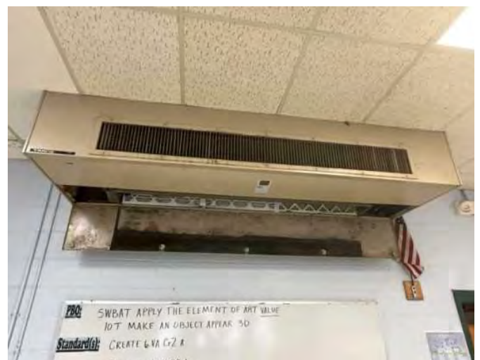
18 - CLASSROOM FAN COIL UNIT
