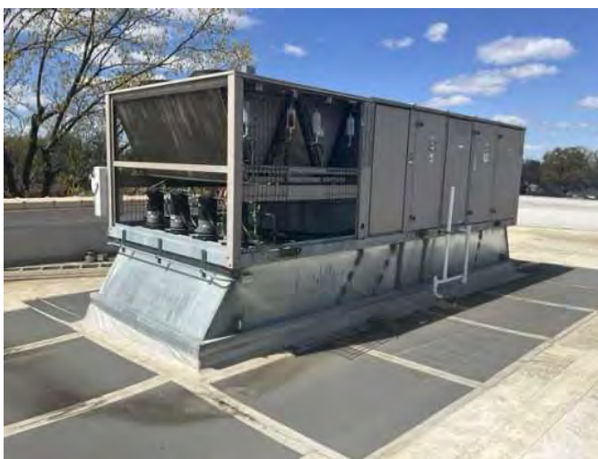
17 - ROOFTOP PACKAGED UNIT
