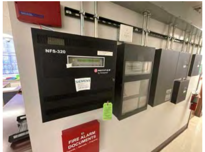
22 - FIRE ALARM PANEL
