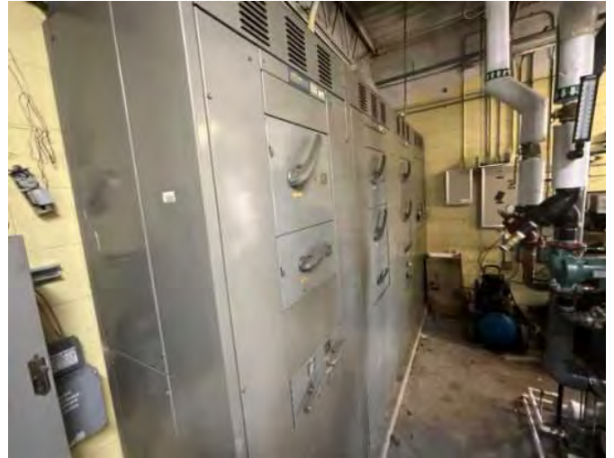
20 - MAIN ELECTRICAL SWITCHBOARD
