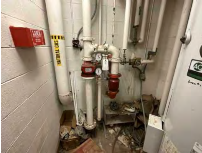
19 - FIRE SUPPRESSION SYSTEM
