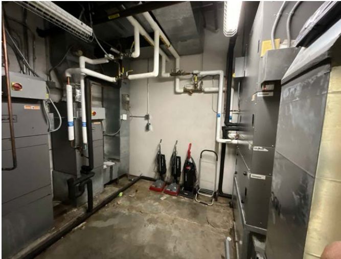
19 - SECONDARY MECHANICAL ROOM
