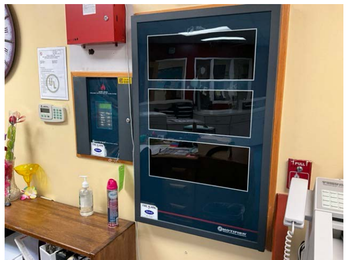
24 - FIRE ALARM PANEL
