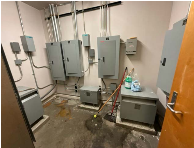
21 - MAIN ELECTRICAL ROOM
