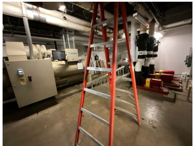
18 - MAIN MECHANICAL ROOM
