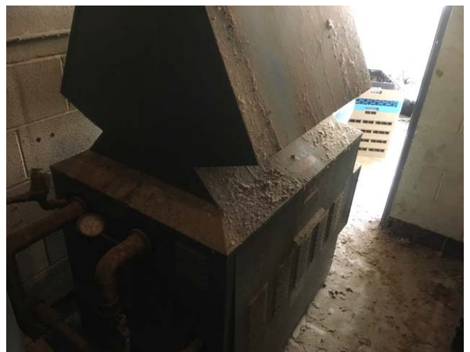
12 - DOMESTIC WATER BOILER
