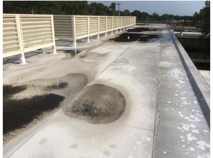
8 - ROOFING, PONDING ISSUE
