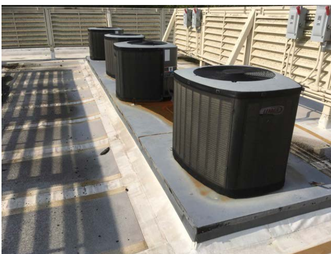
17 - SPLIT SYSTEM, CONDENSING UNIT
