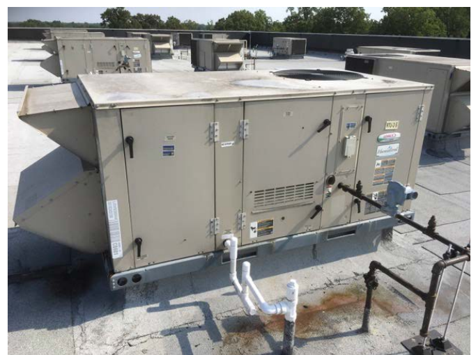
18 - PACKAGED UNIT, RTU
