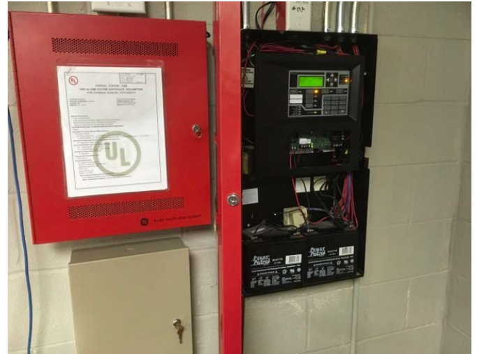
26 - FIRE ALARM PANEL
