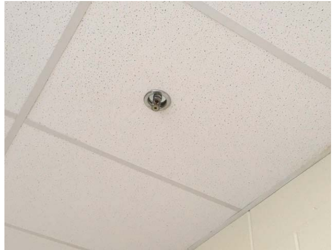
20 - FIRE SUPPRESSION SYSTEM
