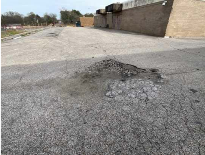
19 - TYPICAL PAVEMENT DAMAGE
