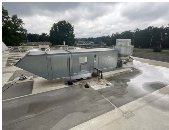
22 - ROOFTOP MECHANICAL EQUIPMENT
