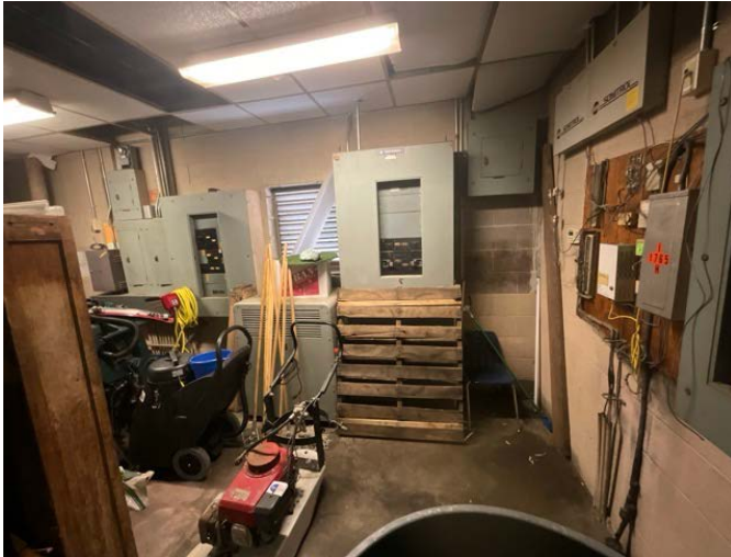
25 - MAIN ELECTRICAL ROOM
