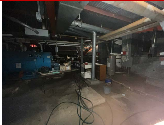
20 - MAIN MECHANICAL ROOM
