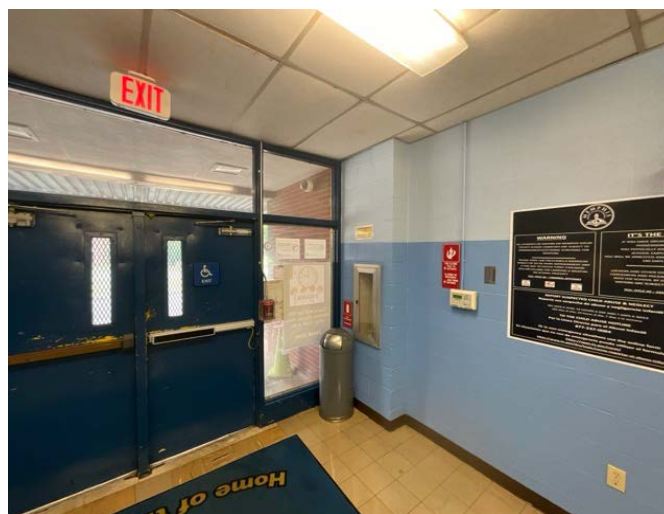
24 - FIRE ALARM DEVICES
