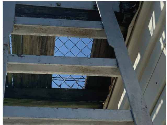
10 - ROOFING MISSING BOARD
