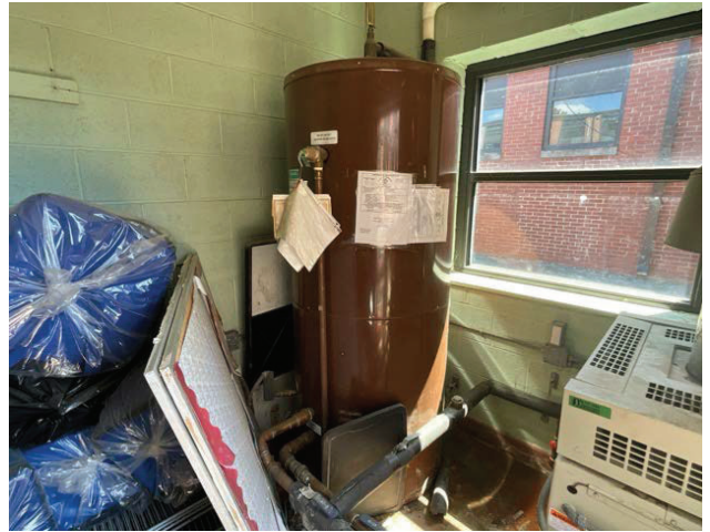
32 - STORAGE TANK W/ BOILER - CLASSROOM
