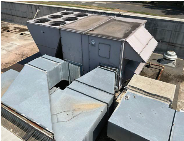
33 - ROOFTOP PACKAGED UNIT - AUDITORIUM
