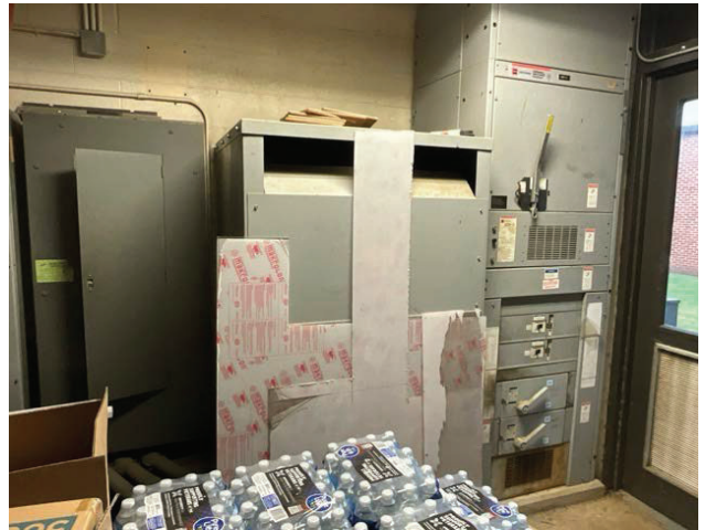
34 - MAIN ELECTRICAL EQUIPMENT - CLASSROOM
