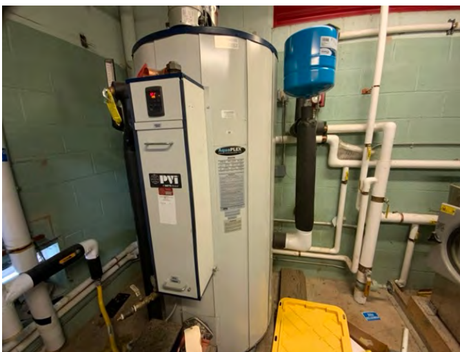
11 - HOT WATER HEATER
