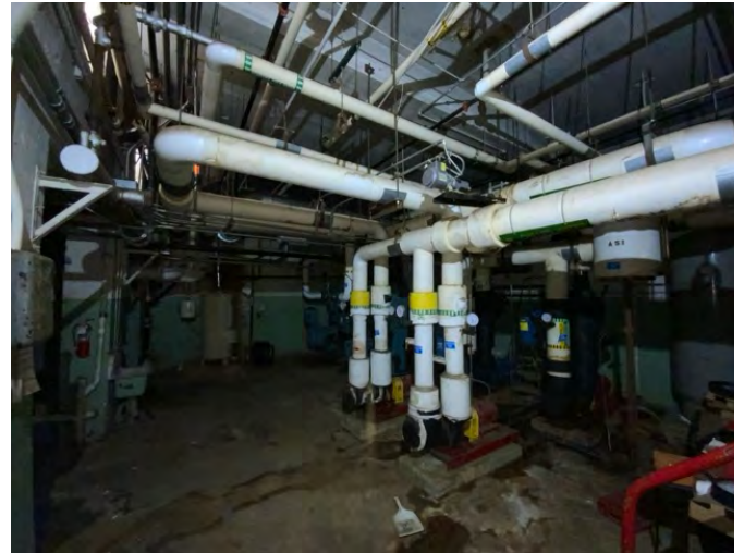
20 - MAIN MECHANICAL ROOM
