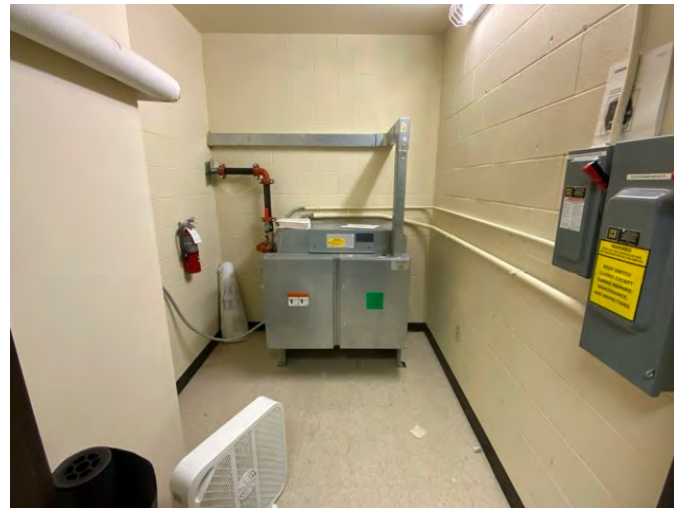
16 - ELEVATOR CONTROL ROOM
