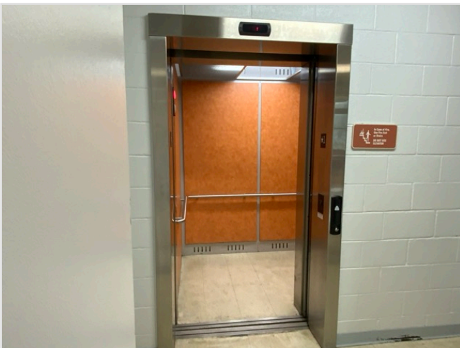
LOBBY LOOKING AT CABS (WITH DOORS OPEN)
