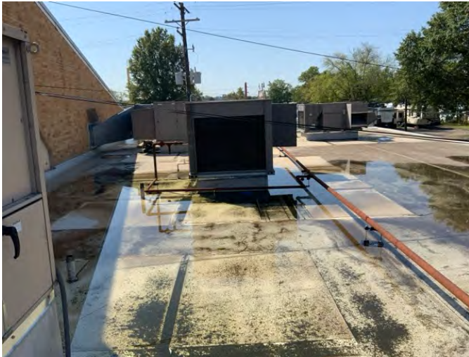
13 - ROOFTOP MECHANICAL EQUIPMENT
