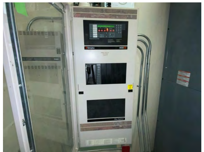
24 - FIRE ALARM PANEL
