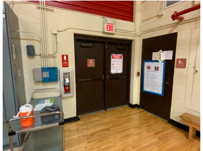
14 - FIRE EXTINGUISHER & ALARM DEVICE
