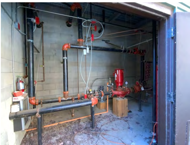
23 - FIRE PROTECTION ROOM
