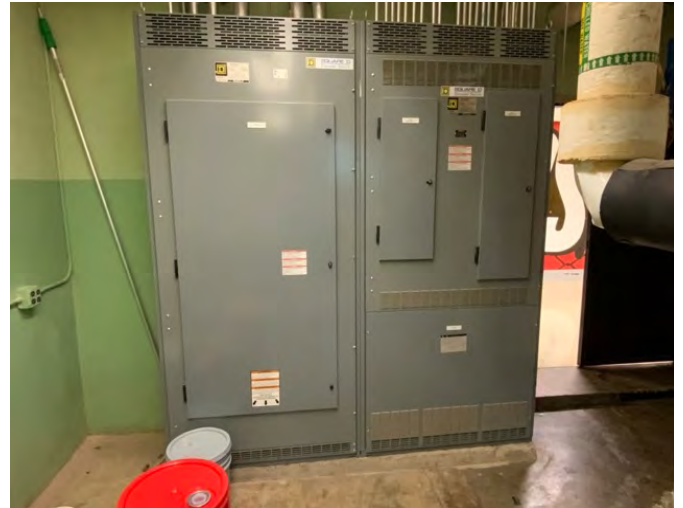
26 - SECONDARY ELECTRICAL ROOM
