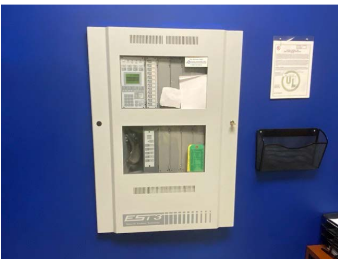
41 - FIRE ALARM PANEL
