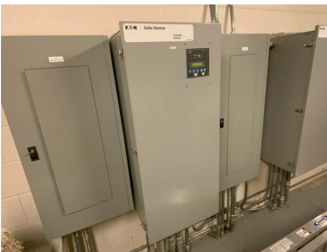
35 - AUTOMATIC TRANSFER SWITCH
