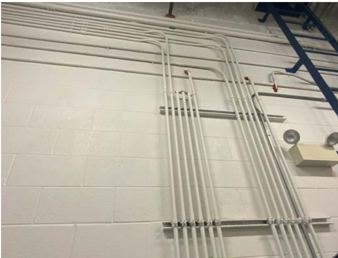
39 - ELECTRICAL SYSTEM WIRING
