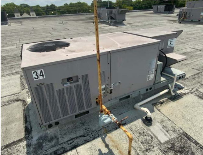
31 - ROOFTOP PACKAGE UNIT
