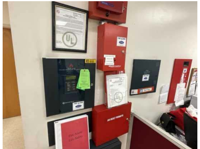
22 - FIRE ALARM PANEL
