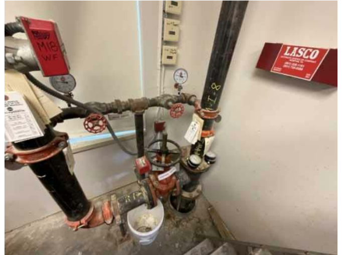
20 - FIRE SUPPRESSION SYSTEM
