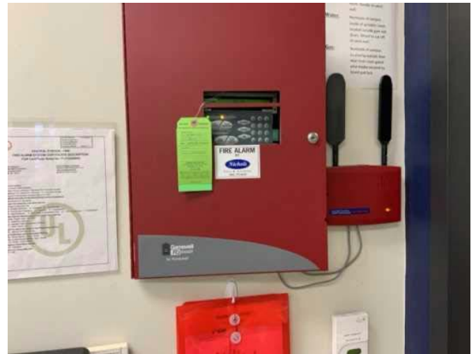
34 - FIRE ALARM PANEL
