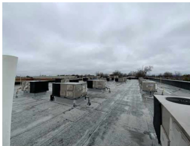
28 - ROOFTOP MECHANICAL EQUIPMENT
