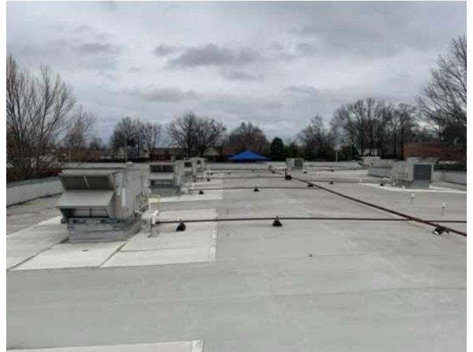
14 - ROOFTOP MECHANICAL EQUIPMENT
