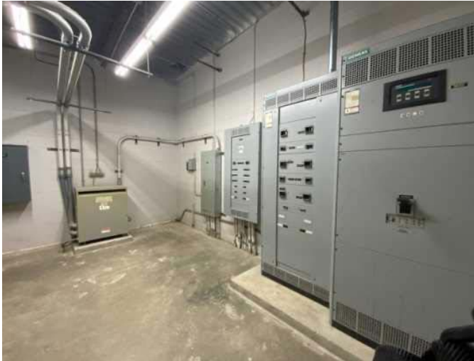
31 - MAIN ELECTRICAL ROOM
