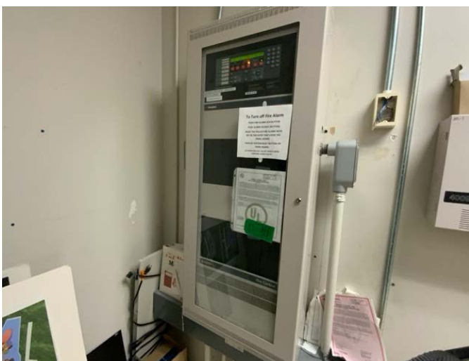
35 - FIRE ALARM PANEL
