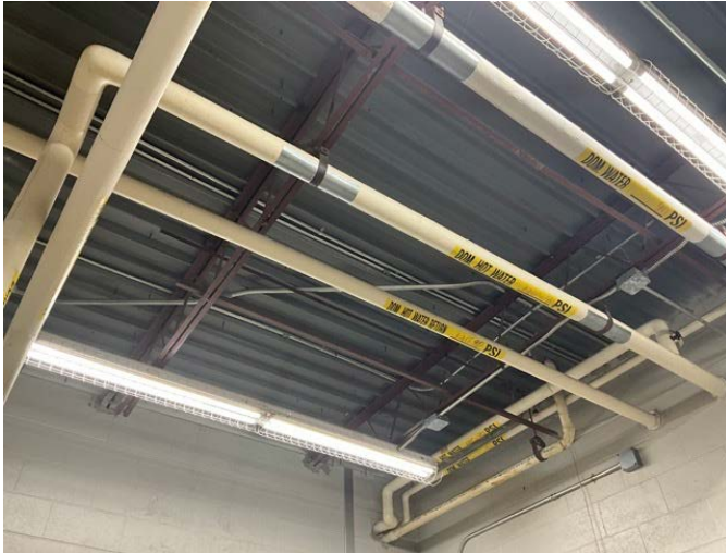
25 - DOMESTIC WATER PIPING
