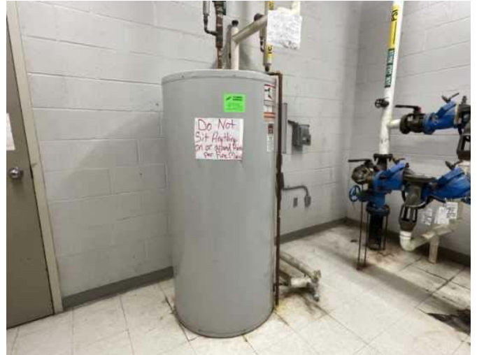
26 - WATER HEATER ANNEX
