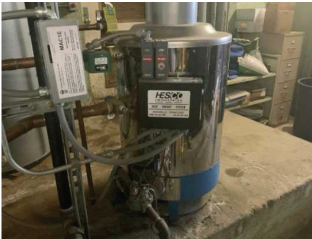
15 - DOMESTIC WATER BOILER
