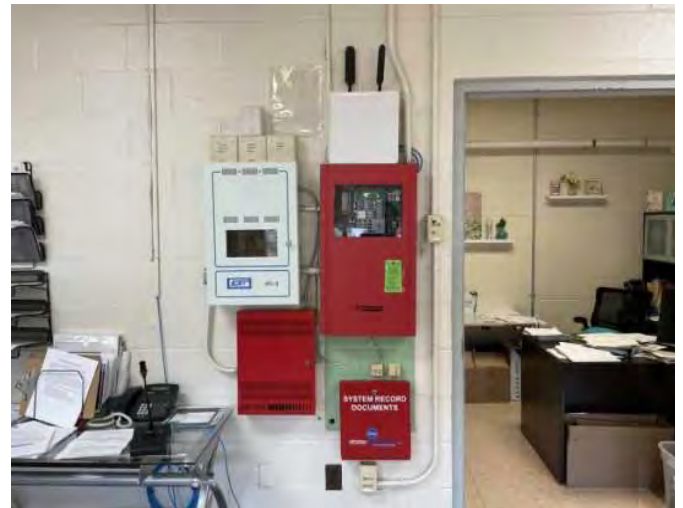
28 - FIRE ALARM PANEL
