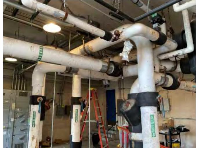
32 - HVAC HYDRONIC PIPING
