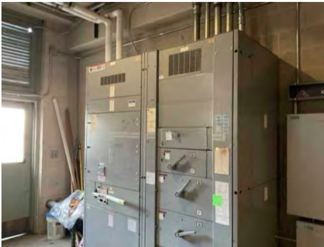
33 - MAIN ELECTRICAL SWITCHBOARD
