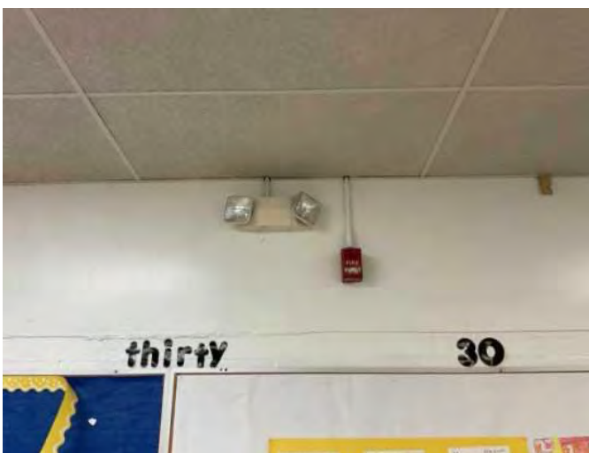
29 - FIRE ALARM SYSTEM
