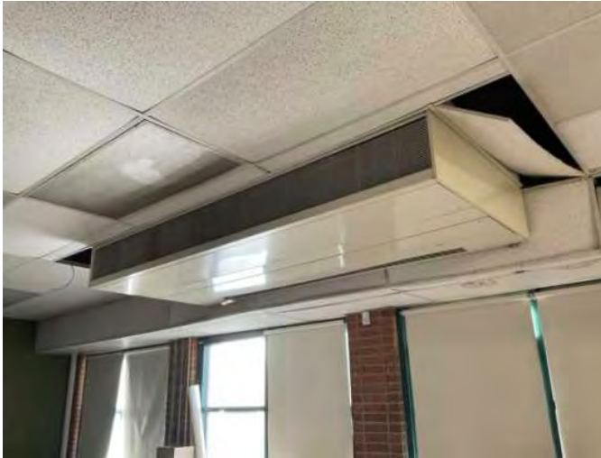
31 - HVAC CLASSROOM UNIT
