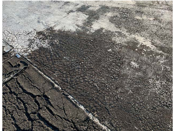
22 - ROOF SURFACE DETERIORATION
