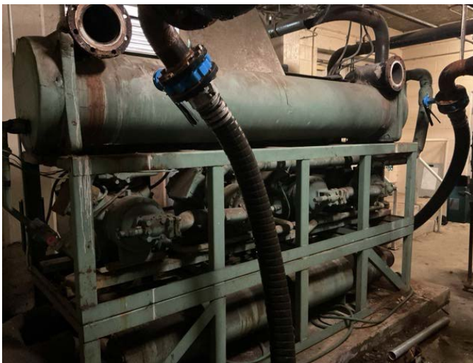
23 - CHILLER (NOT SERVICEABLE)
