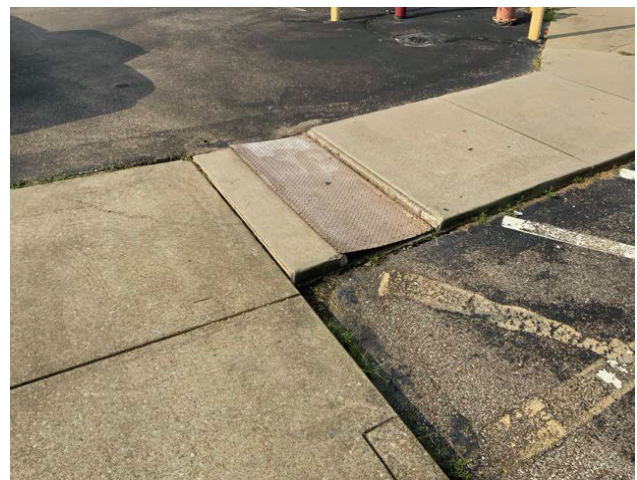
54 - CONCRETE SIDEWALK WITH DAMAGED DRAIN COVER
