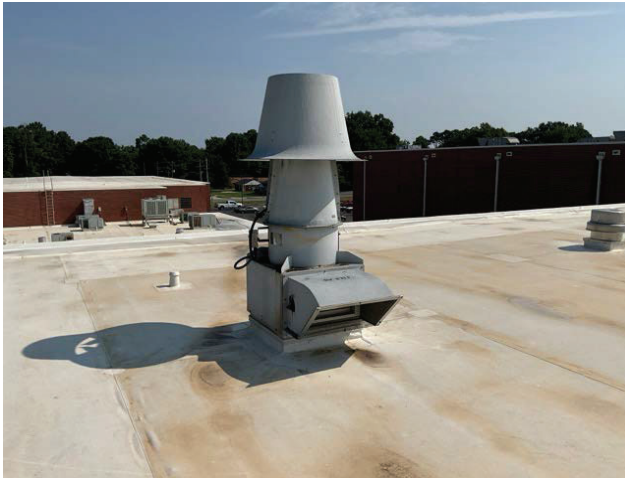
31 - EXHAUST FAN MAIN CLASSROOM
