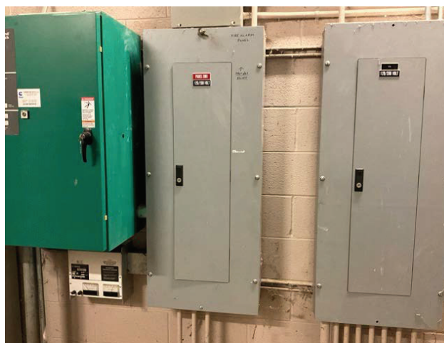
42 - ATS AND DISTRIBUTION PANELS MAIN CLASSROOM
