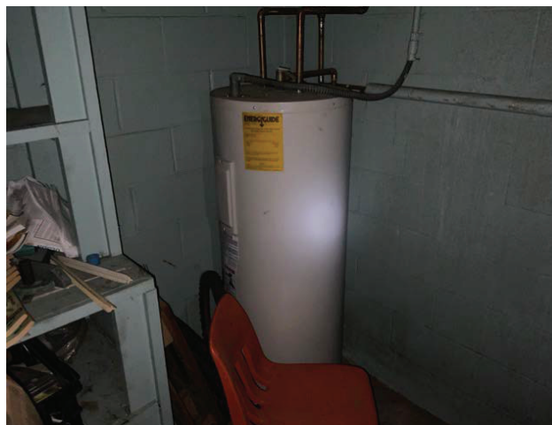
40 - WATER HEATER AUTOMOTIVE SHOP
