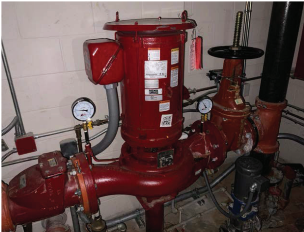
45 - FIRE PUMP MAIN CLASSROOM
