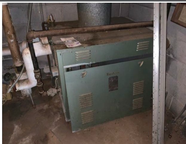
38 – DOMESTIC BOILER GYMNASIUM
