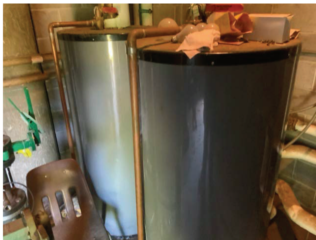
39 – DOMESTIC WATER STORAGE TANKS
