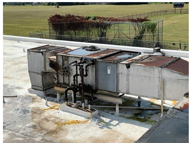
30 - RTU MAIN CLASSROOM
