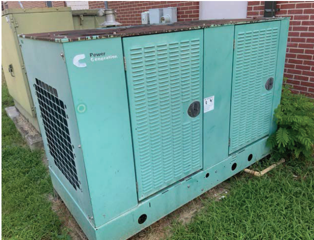
43 - GENERATOR MAIN CLASSROOM
