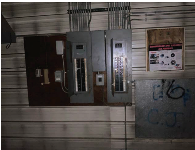
47 - DISTRIBUTION PANEL AUTOMOTIVE SHOP
