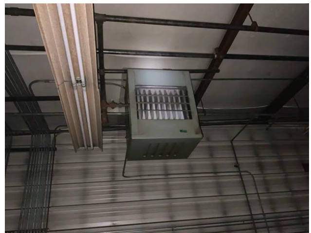
48 - UNIT HEATER AUTOMOTIVE SHOP
