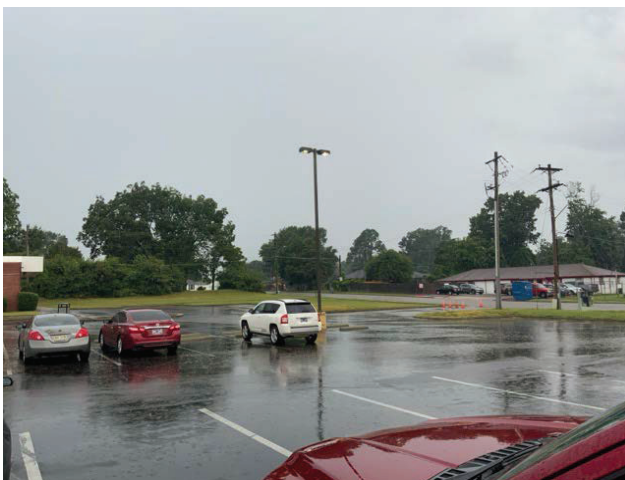
53 - POLE LIGHT FIXTURES
