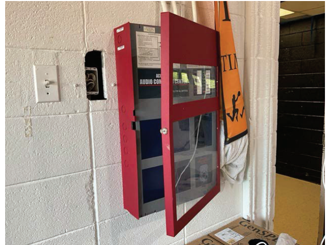
44 - FIRE ALARM PANEL
