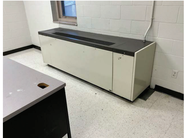
32 - UNIT VENTILATOR MAIN CLASSROOM
