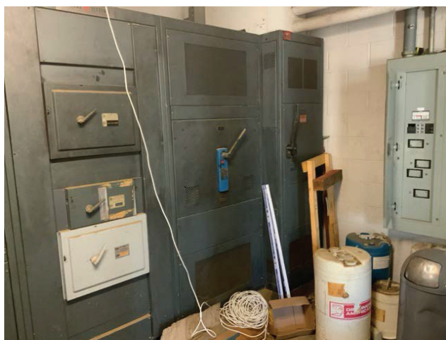
41 - SWITCHBOARD MAIN CLASSROOM
