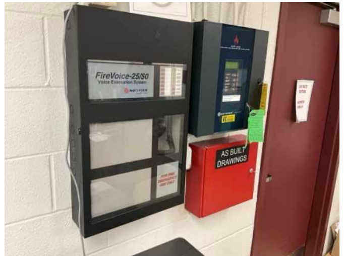
16 - FIRE ALARM PANEL
