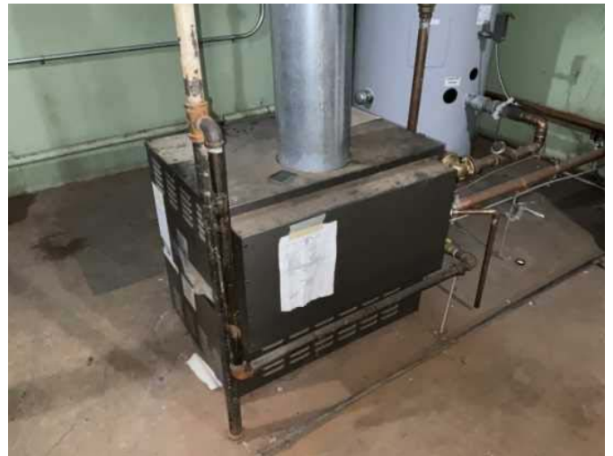
10 - DOMESTIC WATER BOILER
