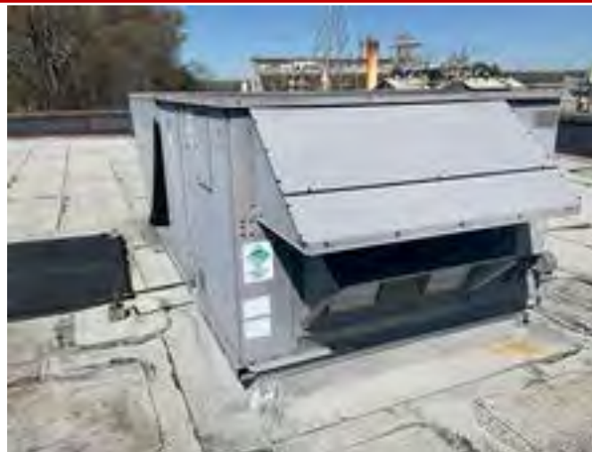
14 - ROOFTOP PACKAGED UNIT
