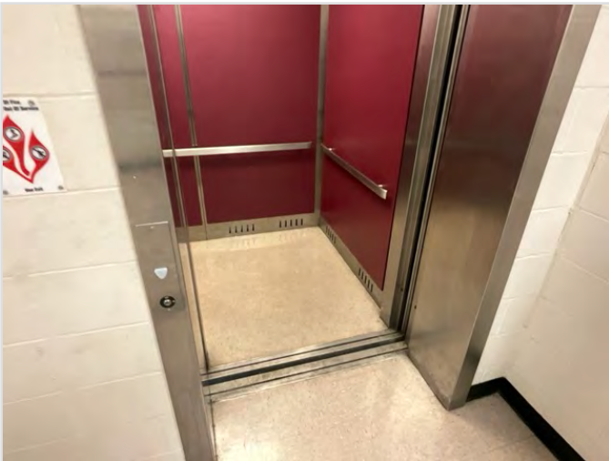
LOBBY LOOKING AT CAB
