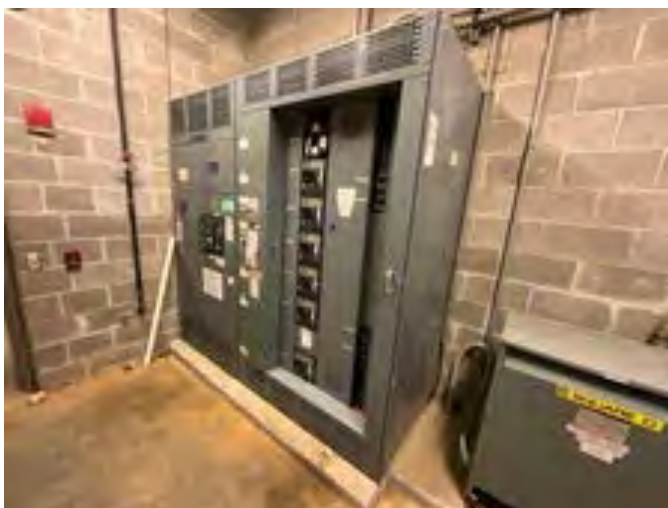
15 - MAIN ELECTRICAL SWITCHBOARD
