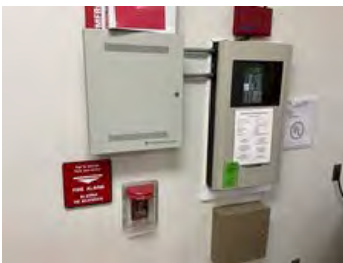
17 - FIRE ALARM PANEL
