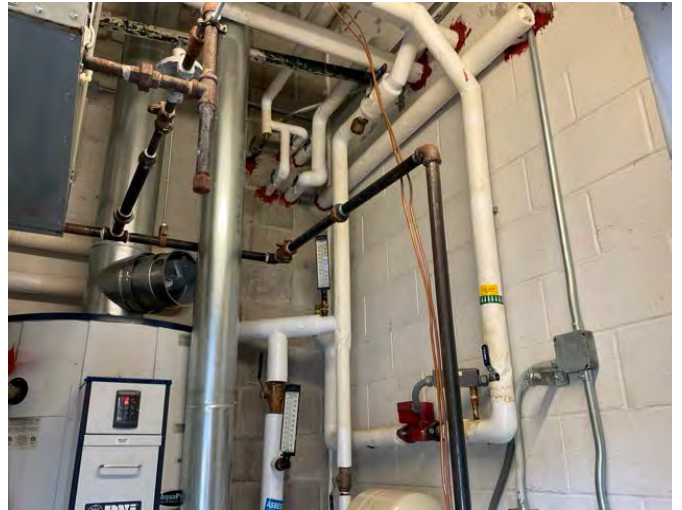
28 - DOMESTIC WATER PIPING
