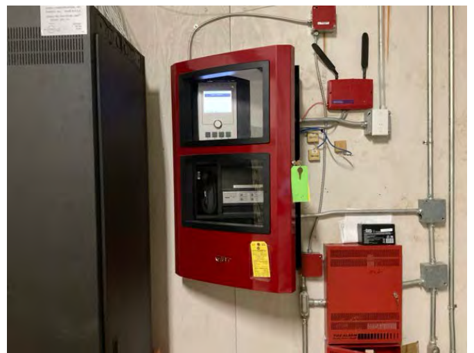
24 - FIRE ALARM PANEL
