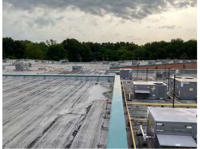
26 - ROOFTOP MECHANICAL EQUIPMENT
