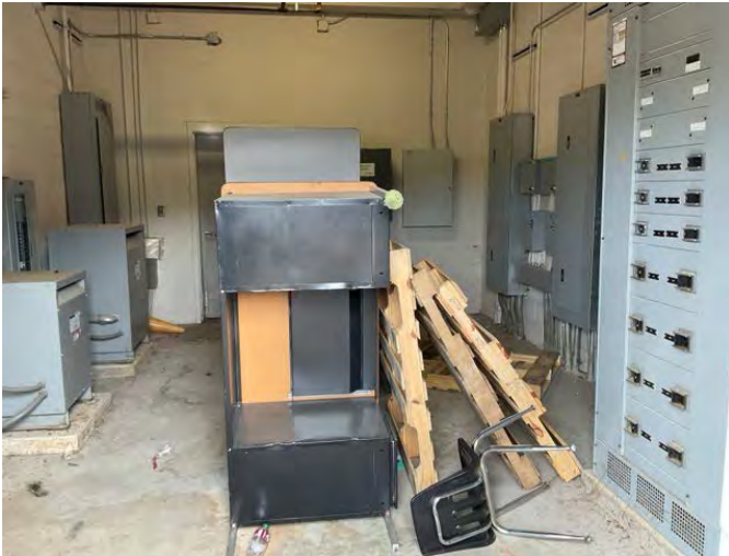
31 - MAIN ELECTRICAL ROOM
