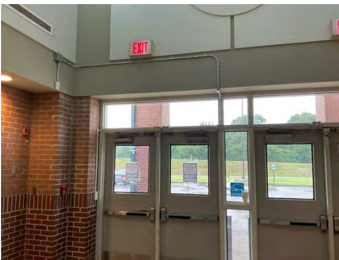
23 - FIRE ALARM SYSTEM
