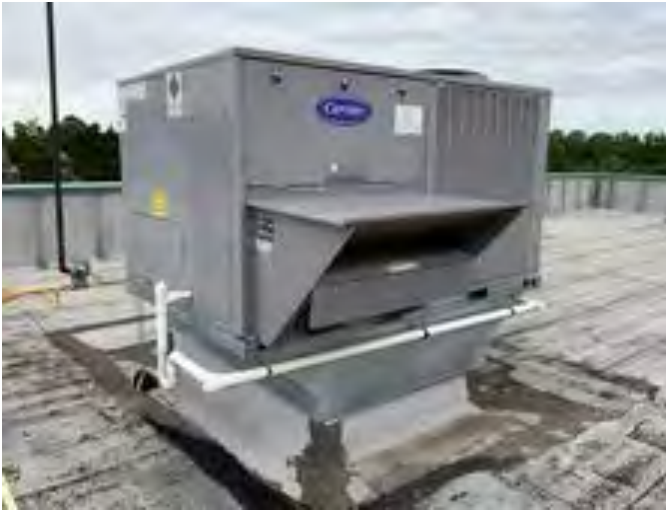
27 - HVAC PACKAGED UNIT
