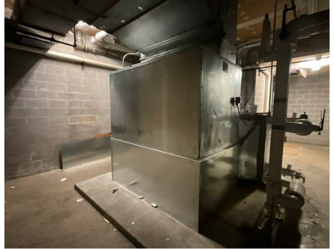
26 - AIR HANDLER UNIT (AHU)
