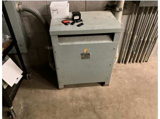
34 - STEP DOWN TRANSFORMER
