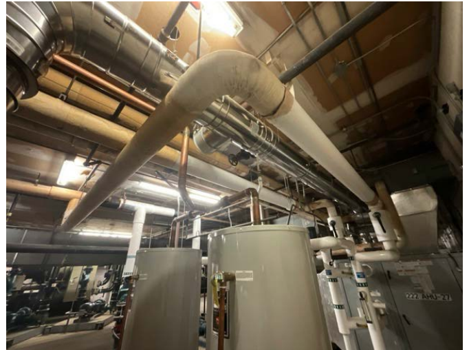
16 - DOMESTIC WATER PIPING
