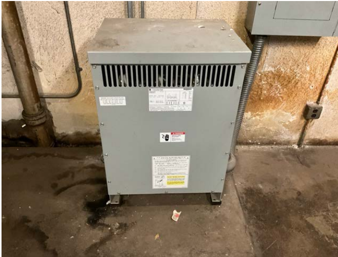
33 - STEP DOWN TRANSFORMER
