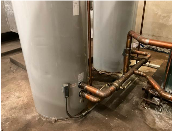
15 - DOMESTIC WATER PIPING
