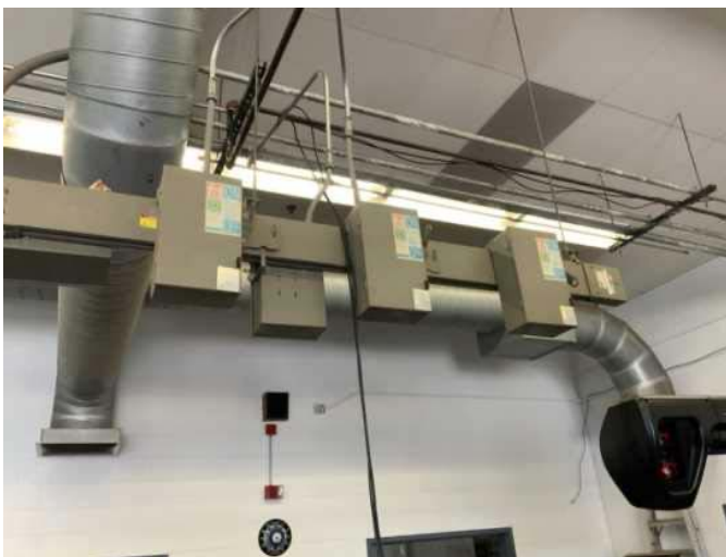
29 - BUS DUCT AND DISCONNECTS
