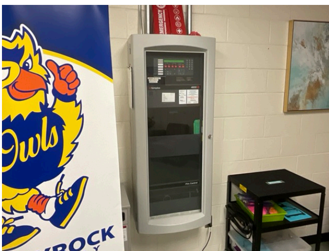
17 - FIRE ALARM PANEL
