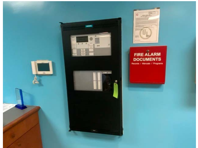
46 - FIRE ALARM PANEL
