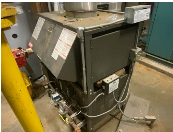
23 - DOMESTIC GAS BOILER
