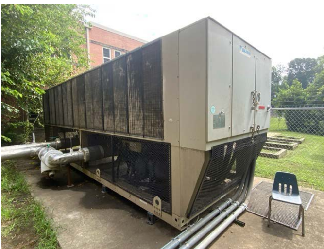
29 - AIR COOLED CHILLER
