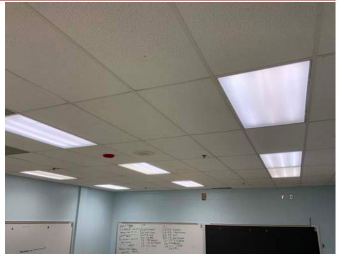
44 - INTERIOR LIGHTING SYSTEM
