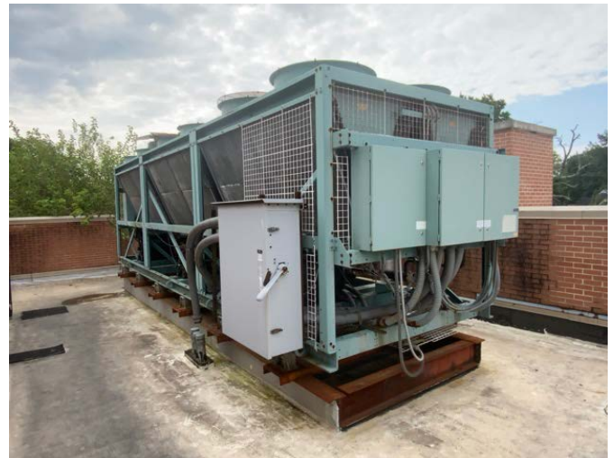
28 - AIR COOLED CHILLER
