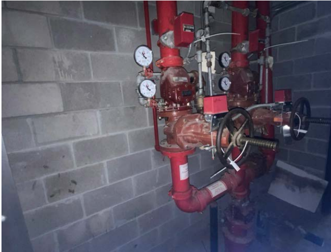
37 - FIRE SUPPRESSION SYSTEM
