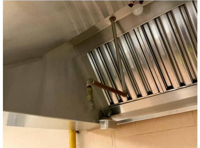
38 - KITCHEN HOOD SUPPRESSION SYSTEM
