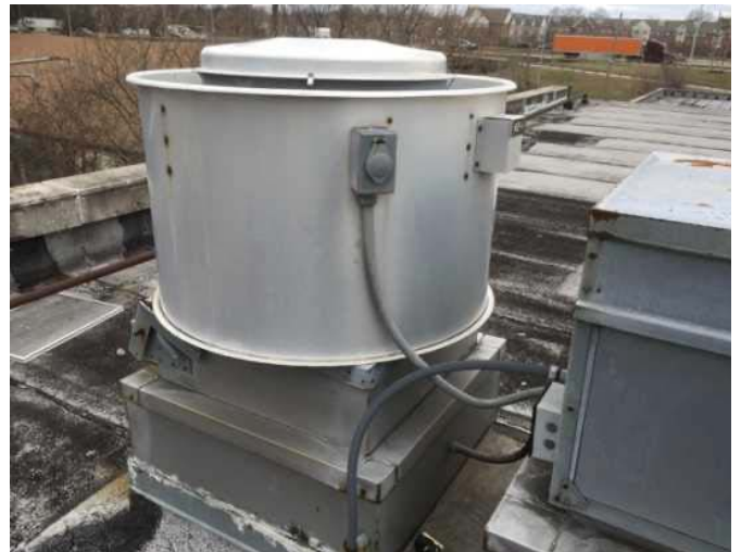
28 - EXHAUST FAN, ROOF
