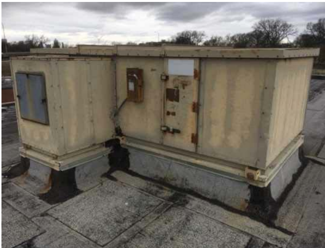
27 - AIR HANDLER, EXTERIOR
