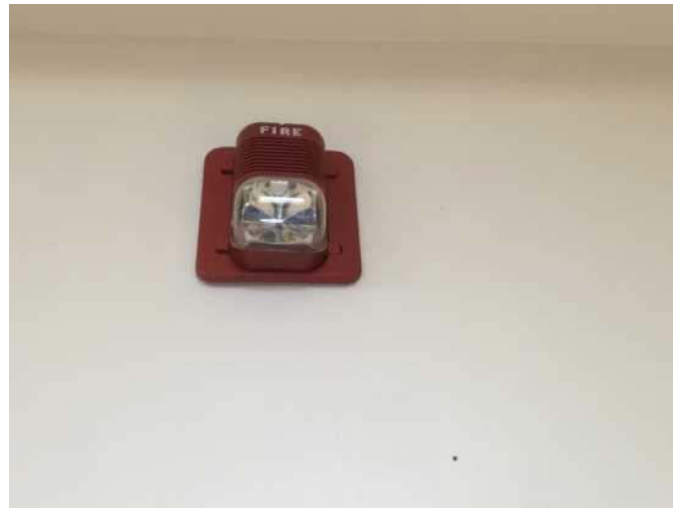
34 - FIRE ALARM SYSTEM
