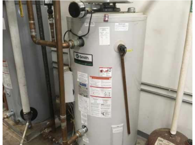
20 - WATER HEATER, GAS
