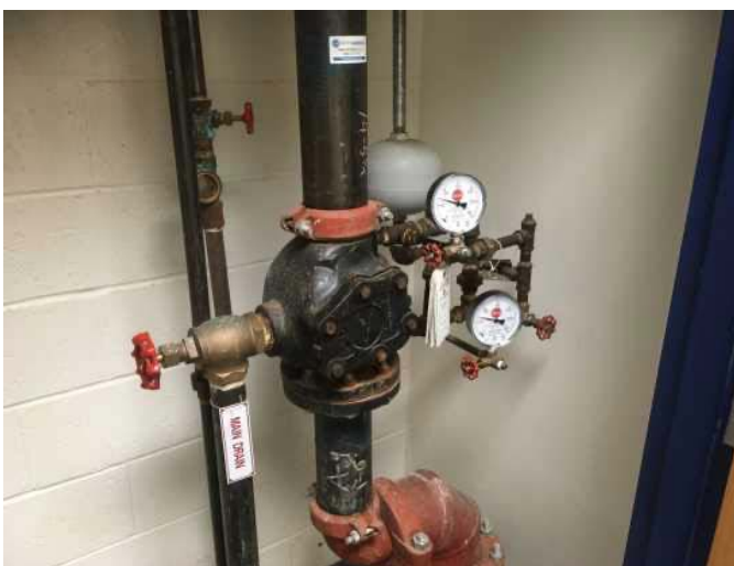
29 - FIRE SUPPRESSION SYSTEM
