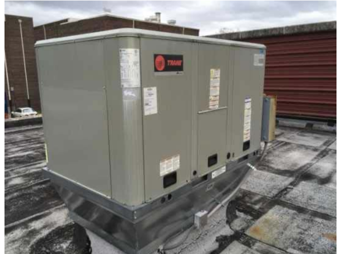
26 - PACKAGED UNIT, RTU
