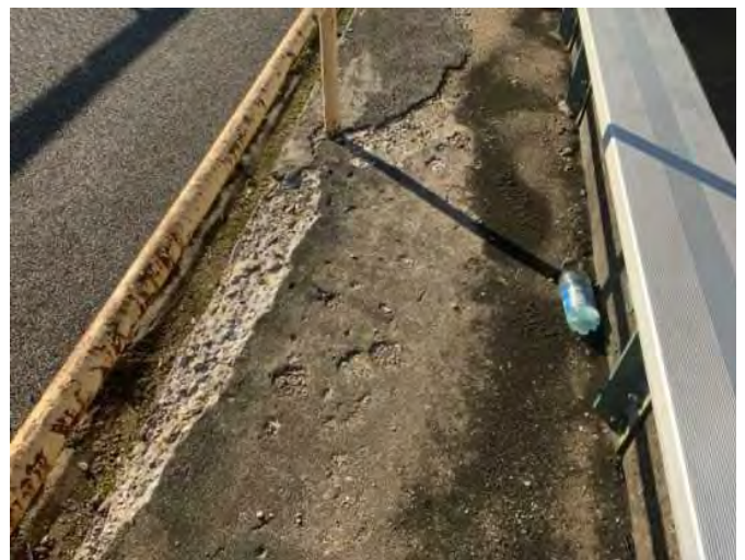
24 - BALCONY STRUCTURE - SPALLING
