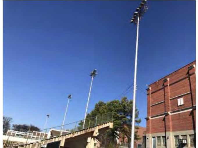
20 - SPORTS FIELD LIGHTING
