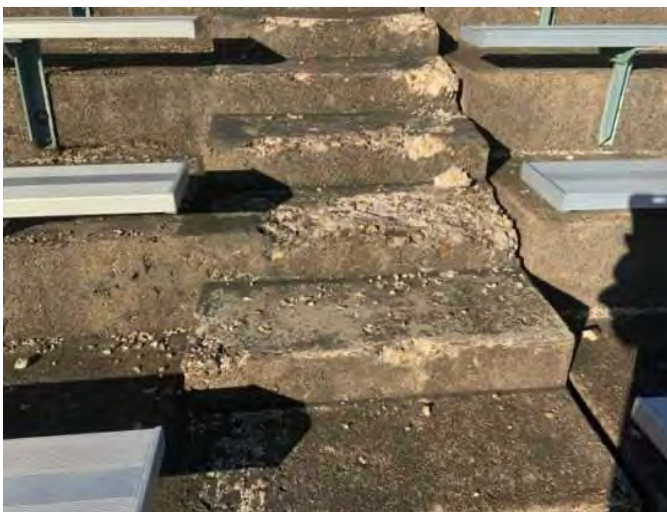
23 - BALCONY STRUCTURE - SPALLING
