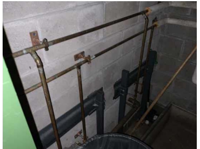
22 - DOMESTIC WATER PIPING
