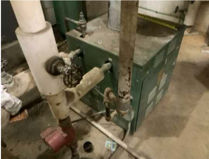
25 - DOMESTIC WATER BOILER
