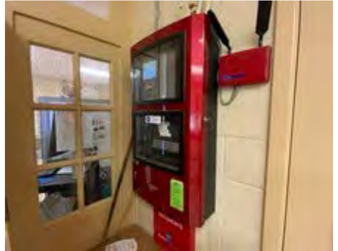
38 - FIRE ALARM PANEL
