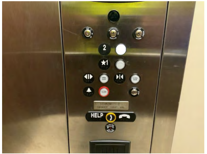
In-cab controls/emergency call panel
