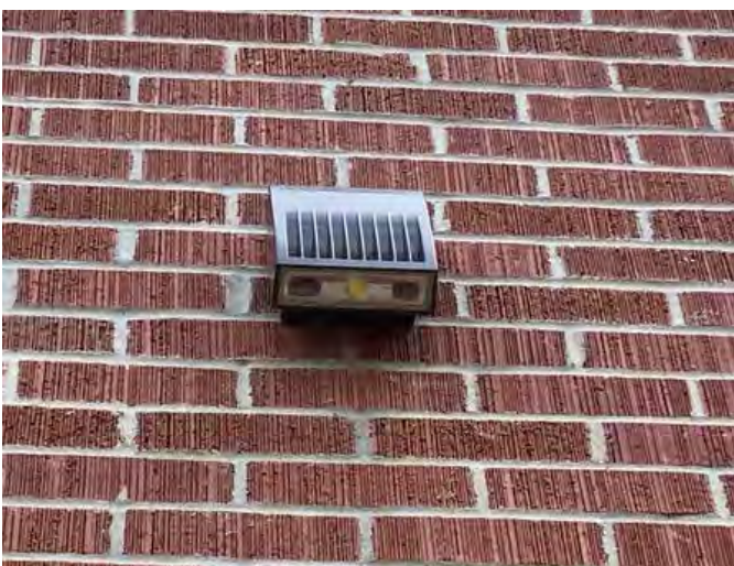
35 - EXTERIOR FIXTURE W/ LAMP
