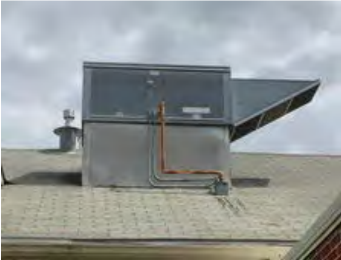
31 - MAKE UP AIR UNIT
