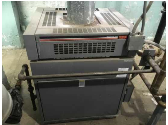
16 - DOMESTIC BOILER, GAS
