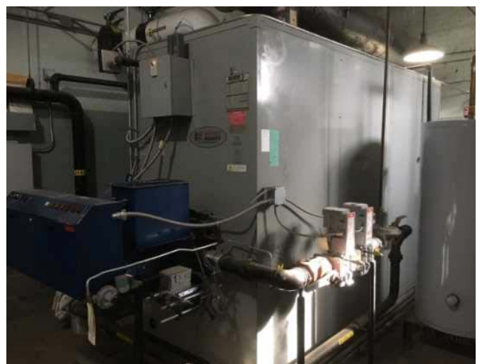
18 - HVAC BOILER, GAS
