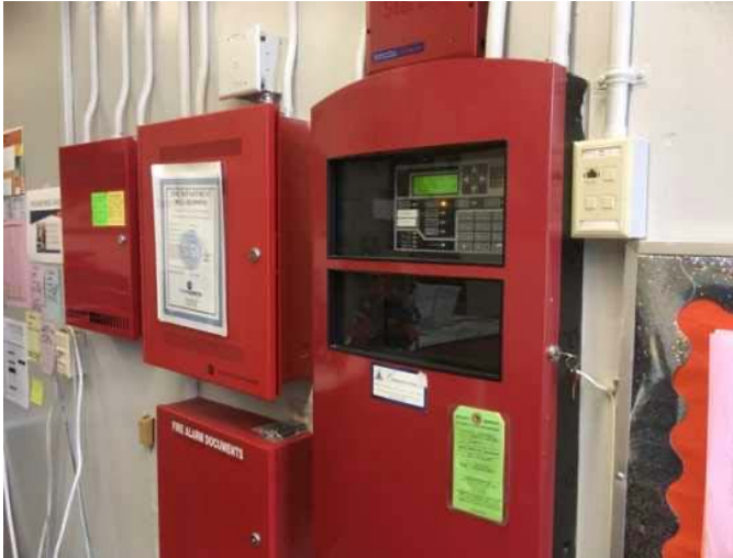
25 - FIRE ALARM PANEL
