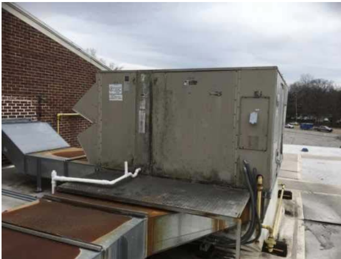
21 - PACKAGED UNIT, RTU
